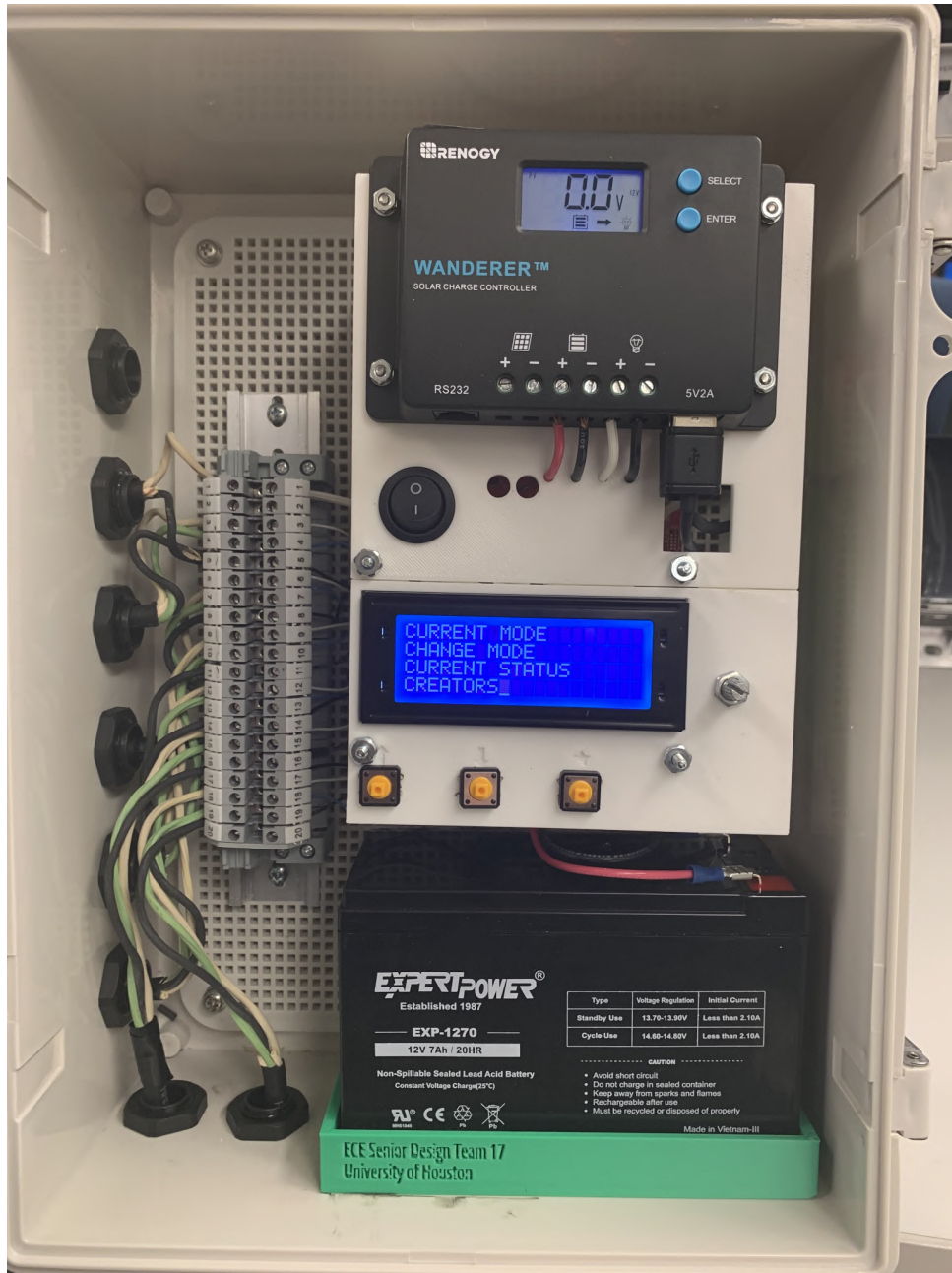
Figure BU: Exterior Wiring coming into the DIN Rail
